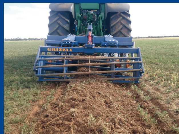
Renovated track after 2 passes – notice the slight mound on track to help shed water
